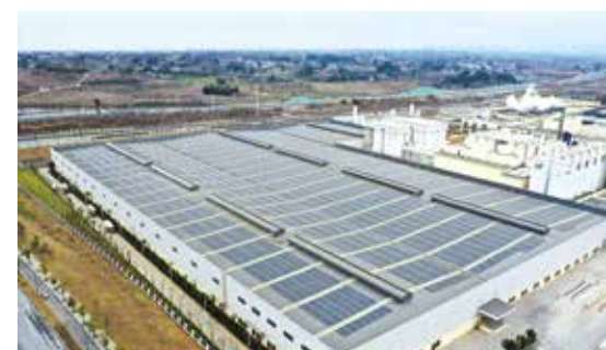
Jushi Chengdu Intelligent Production Base commenced operation of the largest 11.6 MW distributed PV power station in Chengdu.
